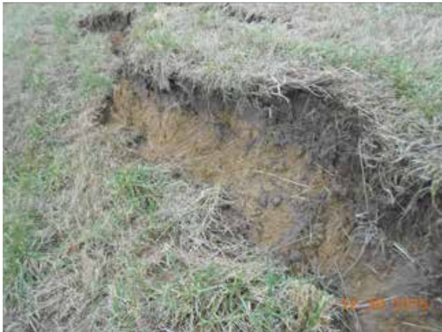
Figure G.2. Photo of 2015 sloughing prior to repairs.
